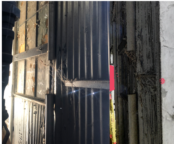
Figure 3: Photo and MiraCAD model comparison of the interior view of the absorption building, depicting a member that was manipulated to meet the demands of the oil and gas piping.
