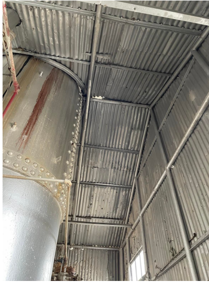
Figure 2: Interior view of the absorption building, depicting the various connections and types of members, alongside the vaulted ceiling and absorption tower.
